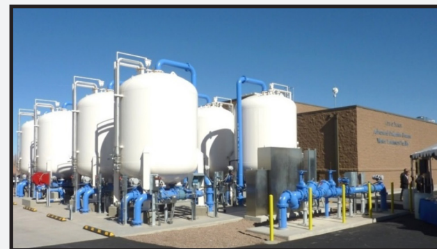
GRANULAR ACTIVATED CARBON TANKS
