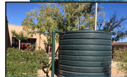
CISTERN OUTSIDE OFFICE BUILDING
